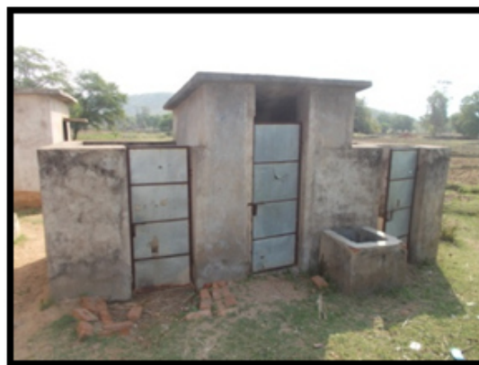
Figure-10: Un used and Damaged condition of Toilet in Mundagaon Primary School.
